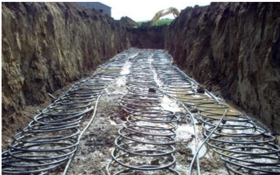
Common ground source field.
